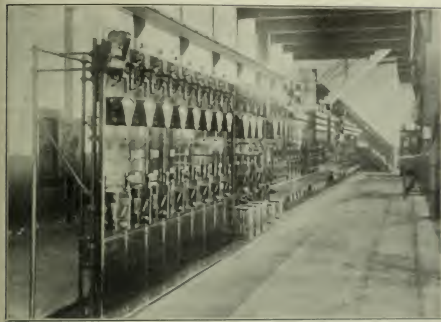
FIG. 11. SWITCHBOARD CONTAINING 57 PANELS
